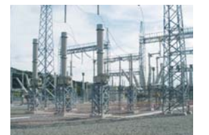
Traction substation for railways
