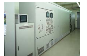
Protection relay & control panel for "Shinkansen Line"
