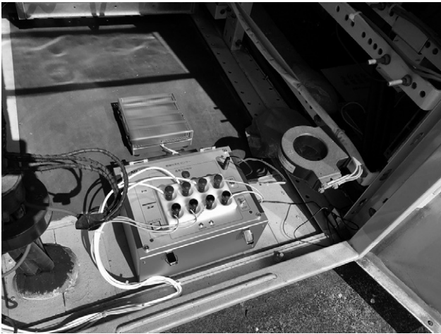
Fig. 7 Installation of an Electrical Insulation Contamination Degradation Trend Sensor Inside a Cubicle
