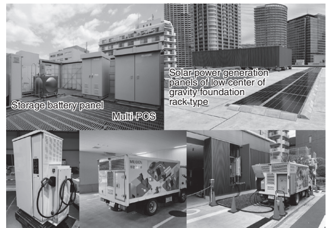
EV charger (to be installed this year) Mobile genset parked on the ground floor parking lot Mobile genset and connector panel for the genset
