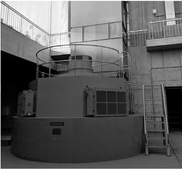
Fig. 13 A View of Completed Generator On-Site
