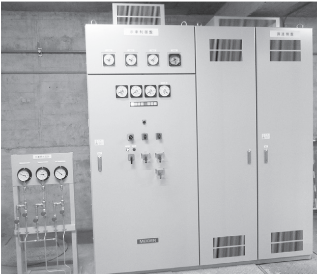
Fig. 4 Hydro Turbine Control Panel and Speed Governor Control Panel
