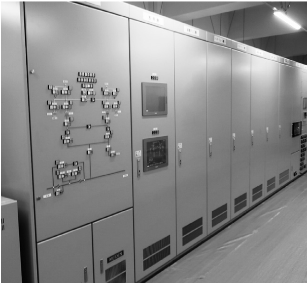
Fig. 11 Supervisory Control Panels Installed at the Omura Depot SS.
