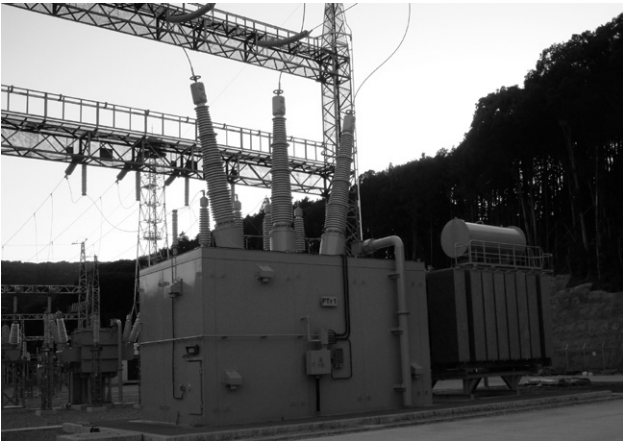
Fig. 4 Roof-Delta Connected Transformer
