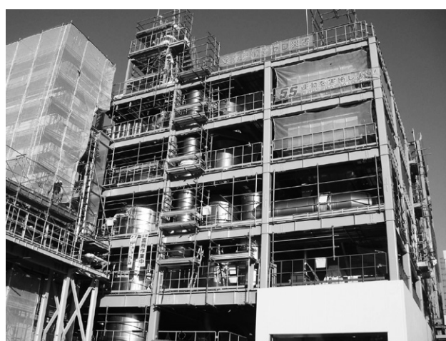
(b) Newly installed
