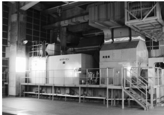
Fig. 5 No.1 Existing 12,500kVA (Gas Turbine) Generator System
