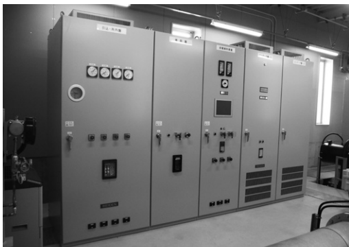
(b) Control panels
