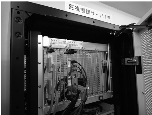
Fig. 2 Plant System Computer, PS6000
