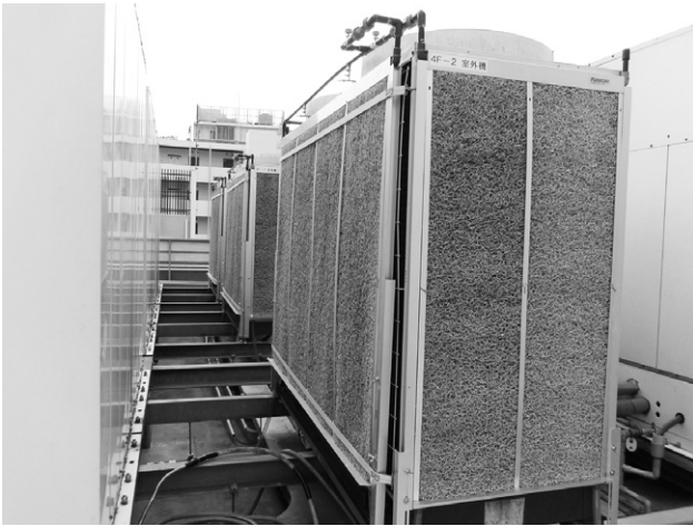
Fig. 4 Example of Indirect Water Spraying Cooler Installations
