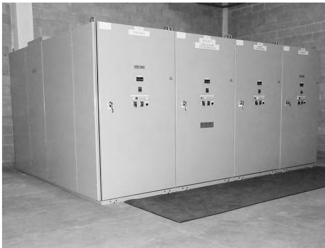
Fig. 3 Outline of 33kV Switchgear Outline of 33kV air insulated switchgear.
