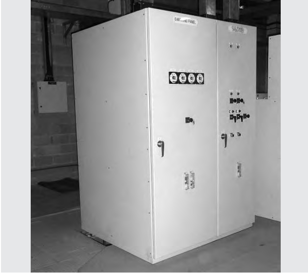
Fig. 6 Outline of Earthing Panel Outline of earthing panel – the DC neutral point is earthed in this cubicle through a grounding resistor.
