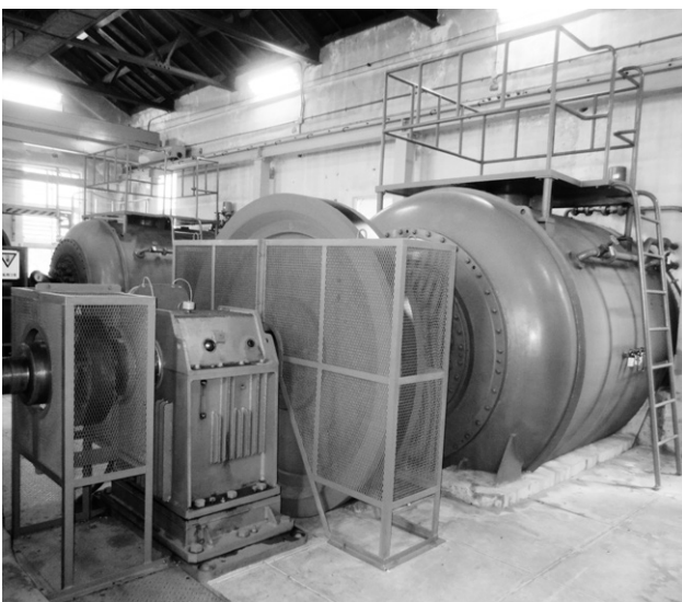
Fig. 2 Existing Generation Facility
