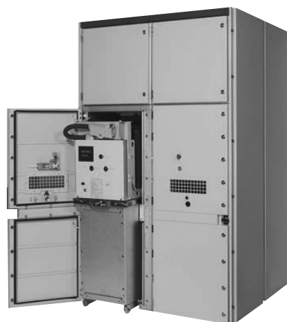
Fig. 7 Track Type VCB and Switchgear
