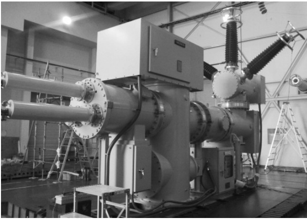
Fig. 3 Situation of Withstand Voltage Test
