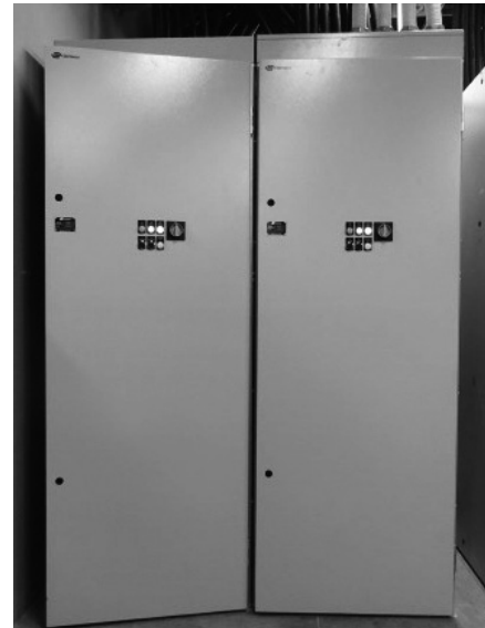
Fig. 11 750V DC Bypass LBS Panel
