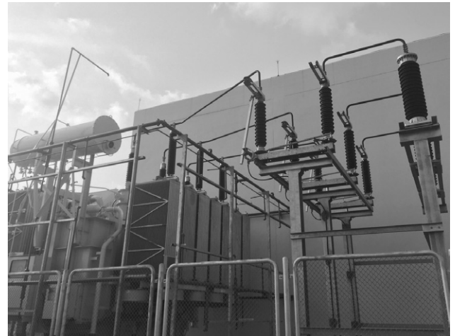
Fig. 5 112/22.8kV Main Power Transformer
