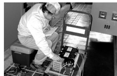
Fig. 4 Example of Testing Executed by a New “Artificial Ground Fault Testing System”
